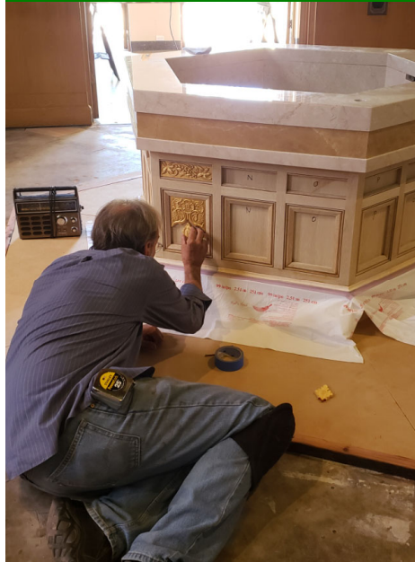
Jim finely tunes the placement of some of the motifs on the Baptismal font. Architectural renderings can't take into account the fineness of some of these details.
