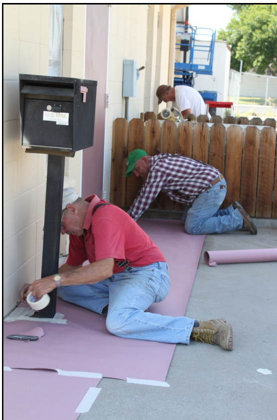
PAINT JOB —Members of St. Patrick's Knights of Columbus recently joined together to help give the exterior of the church a fresh coat of paint. Here Dennis Kathrein, Marty Maffi and Phil Sabatino prepare the north side of the building for its new face. Thank you ♥ to the Knights for their hard work!
